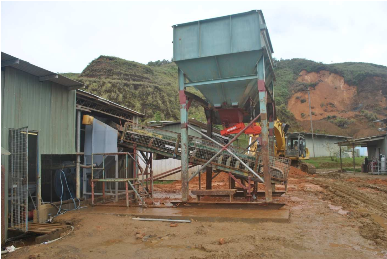
Testing and modifications continued on the newly installed mechanical ball mill feeding plant
